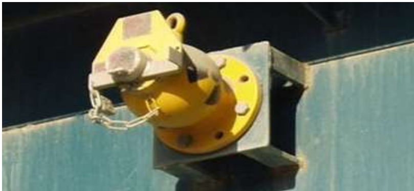
Tank Gauges (Cs-137, 2 to 3 Ci)
